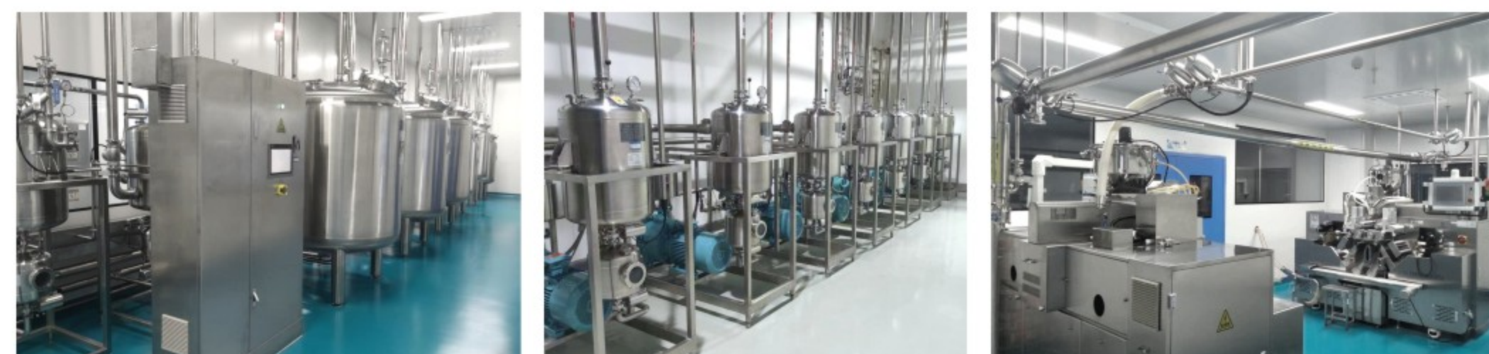
CIP及热水系统 CIP and hot water system
